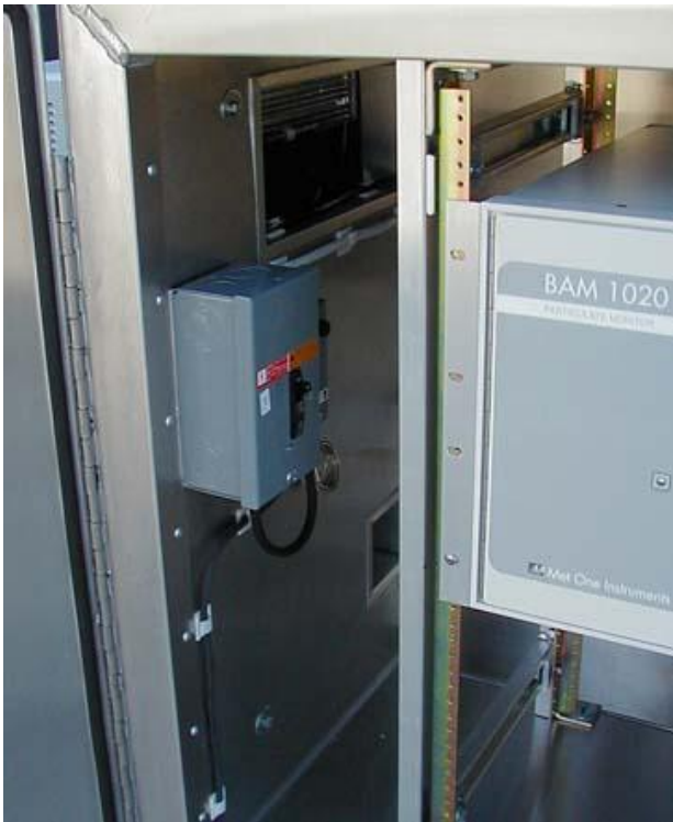
Circuit Breaker Panel Figure 6
